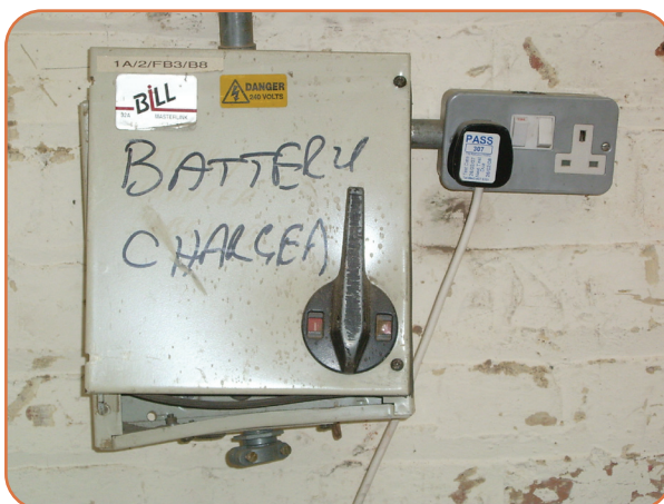
Figure 2-14: Defective electrical equipment. Source: FSTC Ltd.
