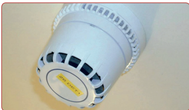
Figure 2-6-47: Smoke detector. Source: RMS.
